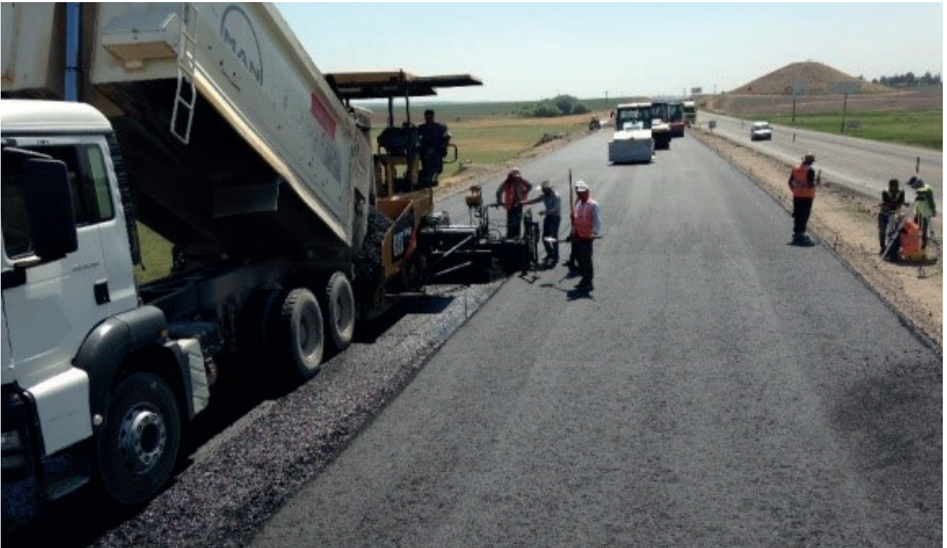
Diyarbakır Bismil Motorway conjunction Project of FERMAK Inc., which is among the companies VEO is cooperating with on projects basis
